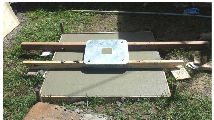
Base concreted in (min. 25mpa) with formwork in place and base elevated 240mm above ground.
